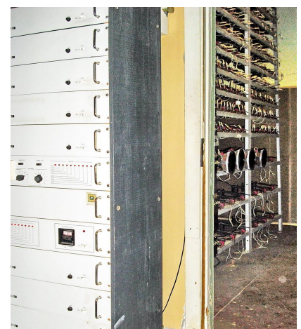
Maximal power testing room
