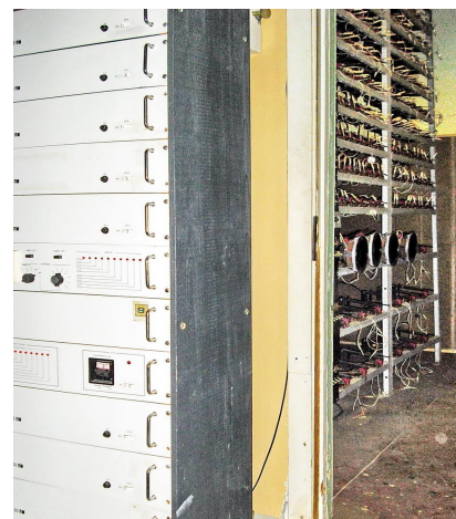
Maximal power testing room
